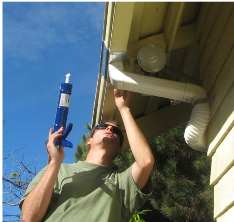
Figure 2.4 SMBRC staff sealing downspout to ensure proper function of the rainwater harvesting system.
