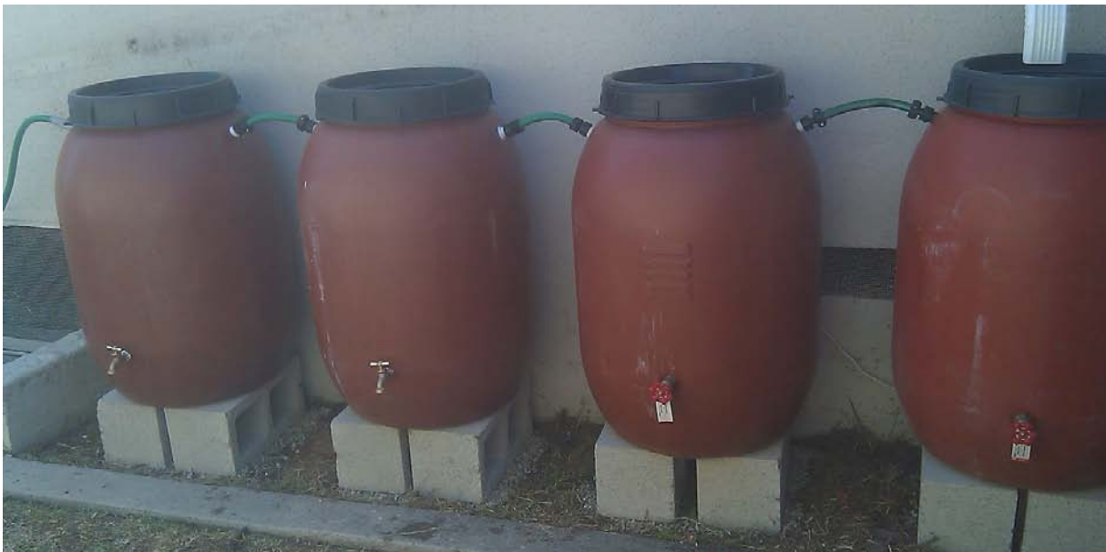
Figure 2.3 Four rain barrels installed in series at a Culver City residence. Flow direction is from right to left (downhill).
