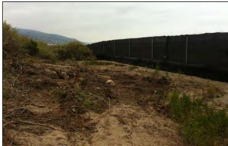
Project area delineated with construction fencing to ensure public safety and delineate work area. Silt fence facilitates animal movement towards adjacent upstream areas and not towards adjacent development (6/14/12).
