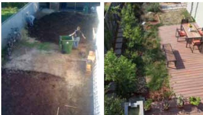
FIG. 5A. The site needed to be modestly re-graded to move runoff away from the house. No soil left the site. The excess soil was used to create a berm, which later became Sage Hill.
