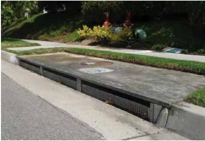
FIG. 6. Curb grate installed at a catch basin opening in the drainage area.
