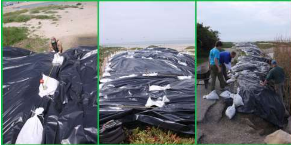
Left: staff suspends sandbags from stakes and lines to hold the plastic sheeting in place on a steep slope. Middle and right: finished sections.
