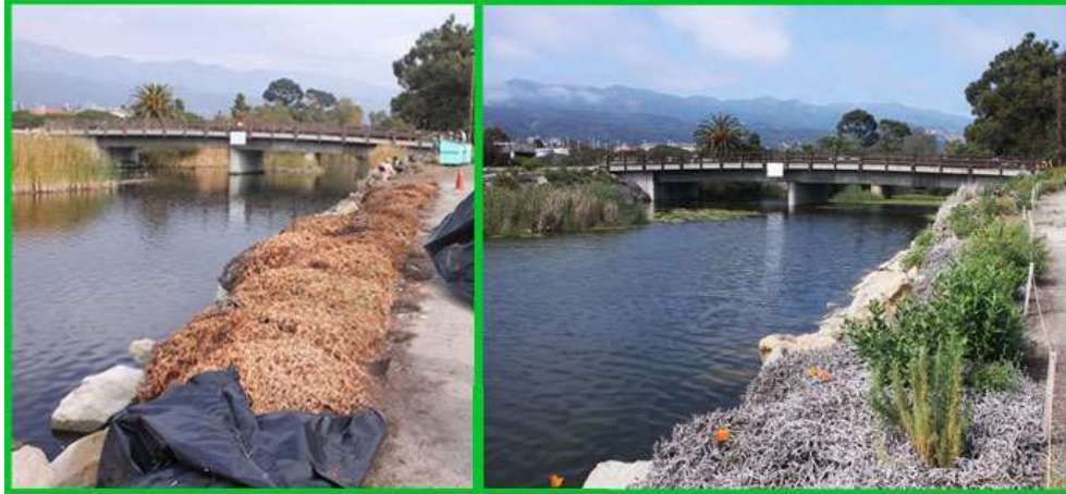
Project site (looking north) after removal of plastic sheeting and initial installation of native plants.
