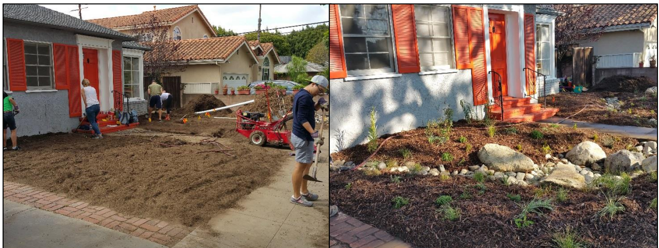
Figure 6. (left) Before: volunteers help remove turf roots, 5/21/2015; (right) After: final day of installation, 4/24/2015.
