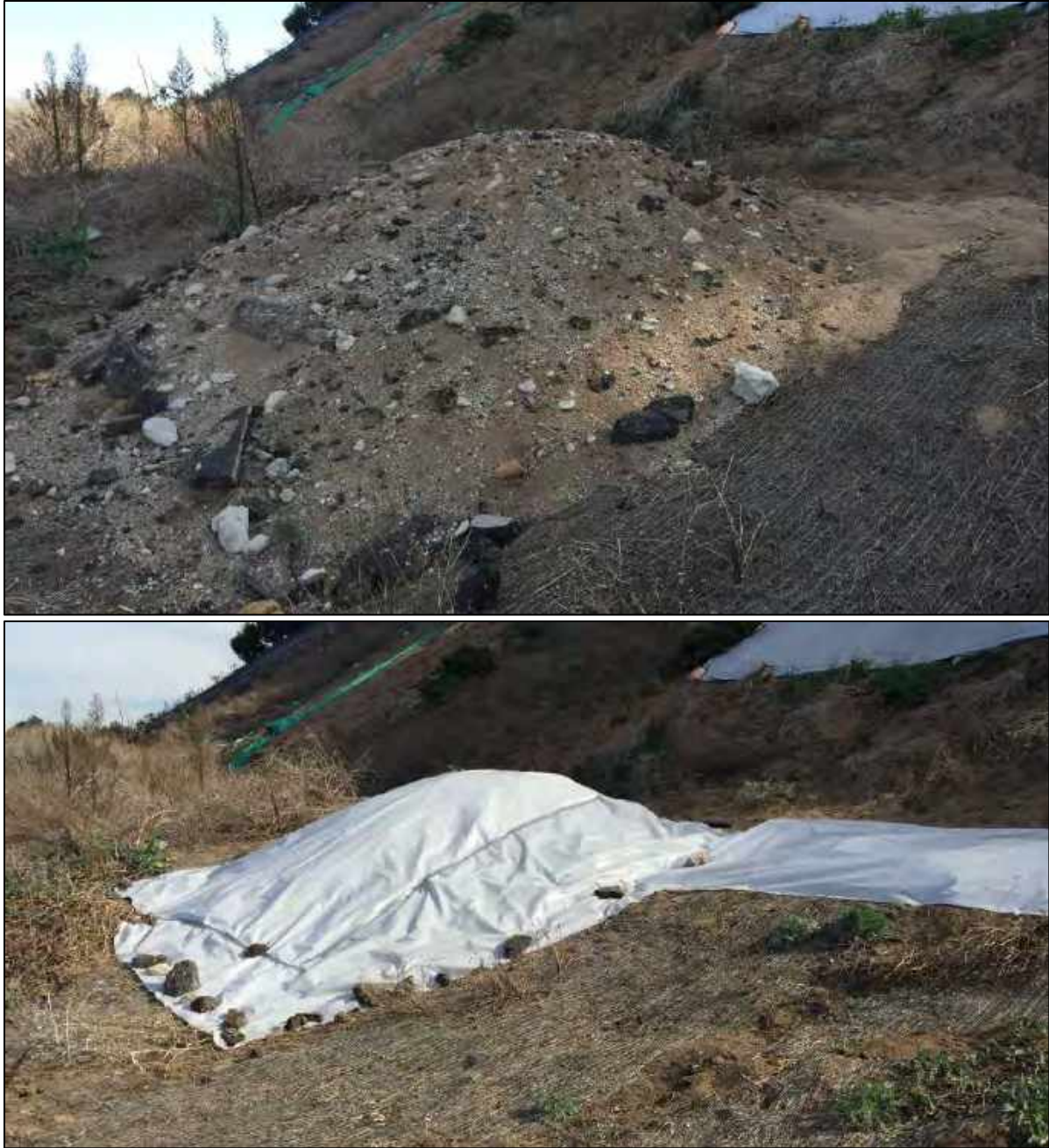
Figure 35. Photographs taken of one of the dumped sediment and trash piles in the restoration area before being covered (top) and after (bottom) (26 November 2019).
