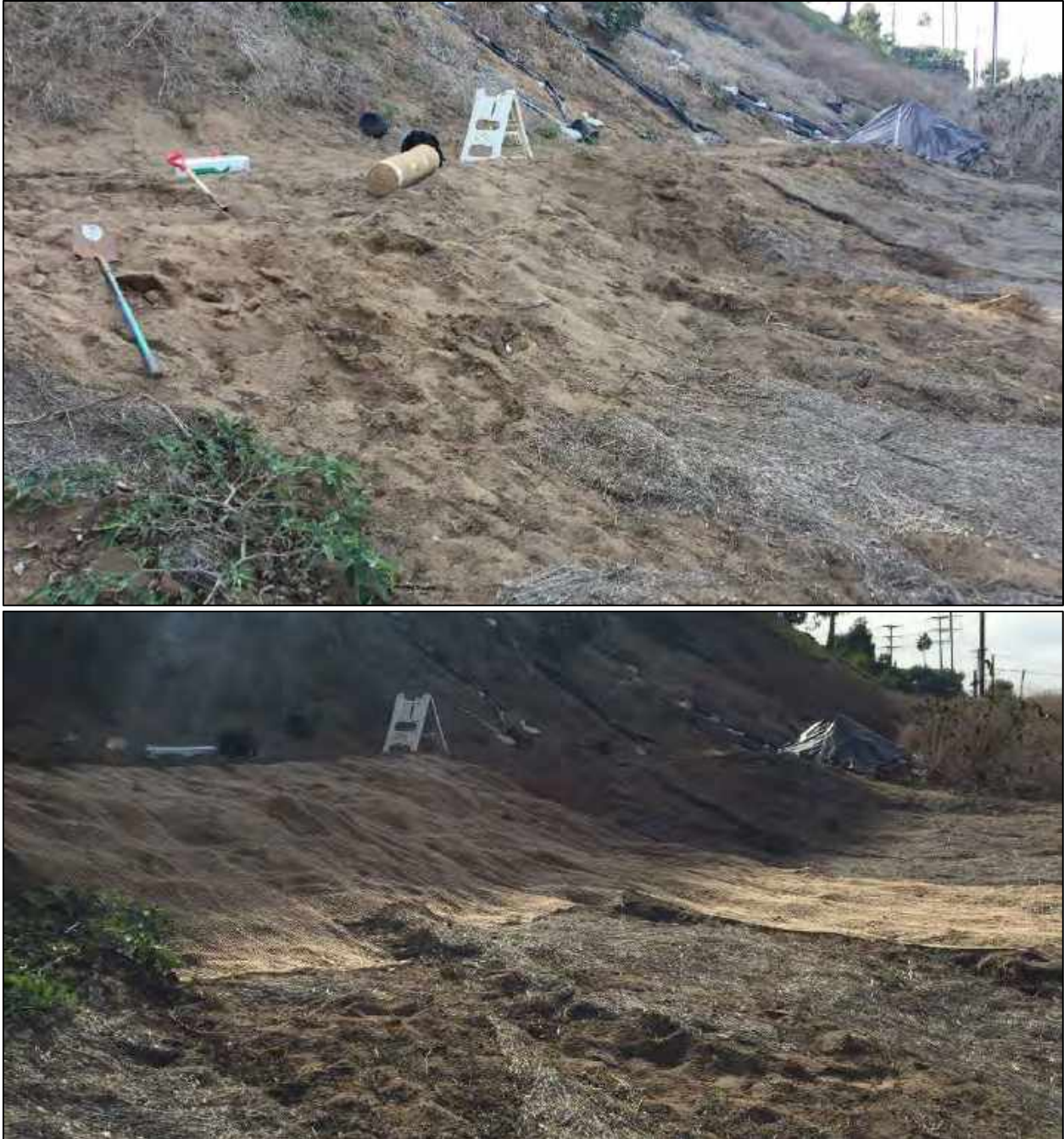
Figure 34. Photographs taken of the impacted area of the hillside with disturbed soils and tracks before emergency measures were taken (top) and after erosion control mats were placed (bottom) (26 November 2019).
