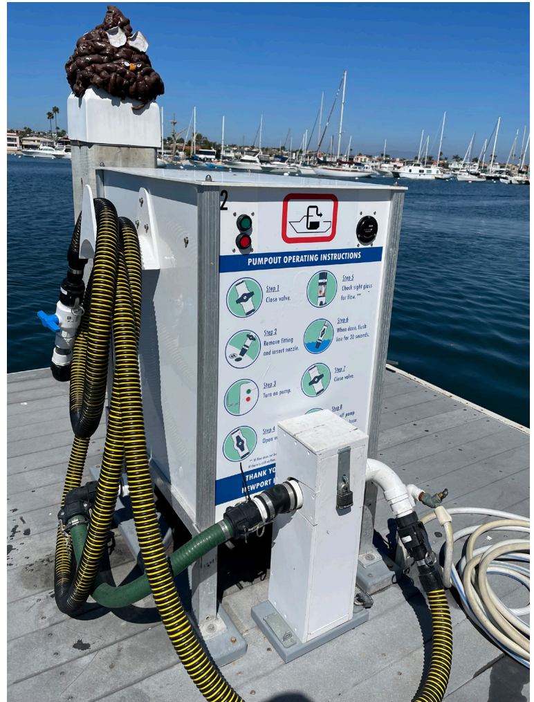
One of the five pumpout units in Newport Beach equipped with the new Particle Separator device.
