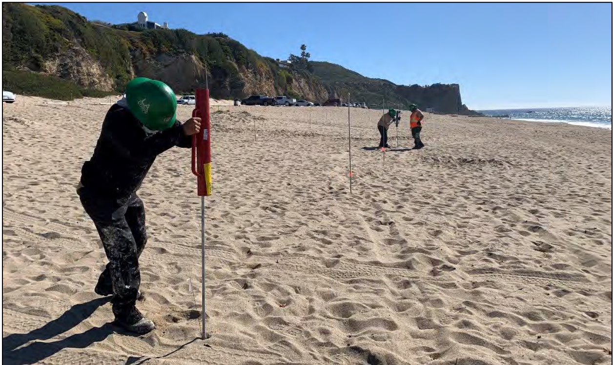
Figure 10a. LACC crew members pounding in posts to delineate the Point Dume project boundary (5 February 2021).
