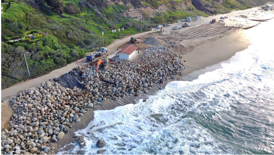
Figure 4. Photo of 2023 after heavy winter storms and mitigation with rip-rap. Photo courtesy of LA County Beaches and Harbors.
