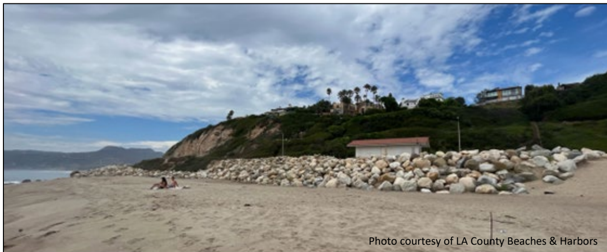
Figure 11. Photo of the transition area between Westward and Pt Dume Beaches, showing the narrow beach and newly installed rip-rap after the 2023 Winter storm damage.
