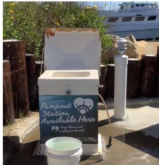
Gravity-drained dump station in Santa Barbara Harbor Photo by TBF
