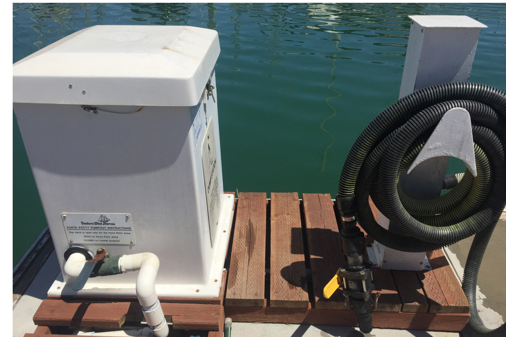
Motorized dump station requiring the manual opening of its ball valve for drainage Photo by TBF
